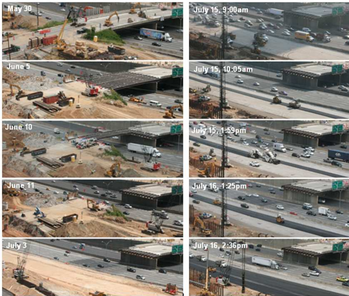
Figure 6 Bridge demolition by daily progress (left), Pavement process by the minute (right)
