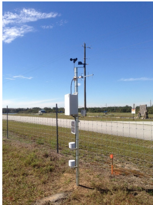
Figure 3-2 Fog monitoring station
